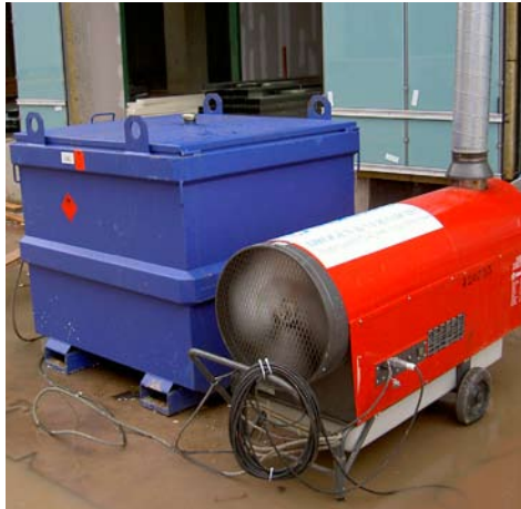
Small construction heating.
