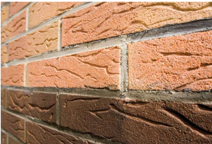
A smoke damaged external wall that has been cleaned using DeKonPeel®.
