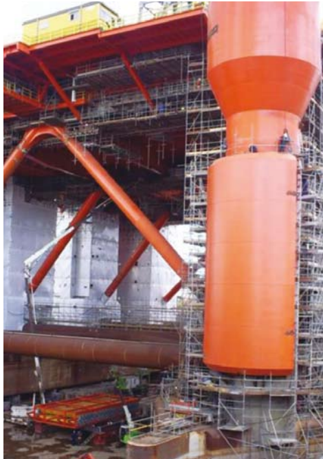
An oil rig being painted. The dehumidifiers protect the steel pillars from corrosion during blasting and before painting.
