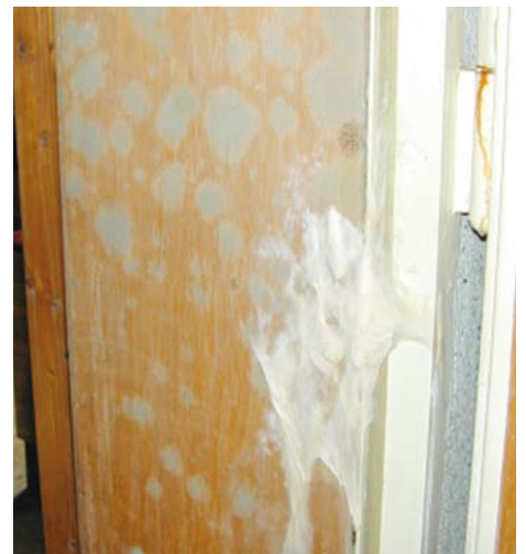
Mildew on door after water damage.
