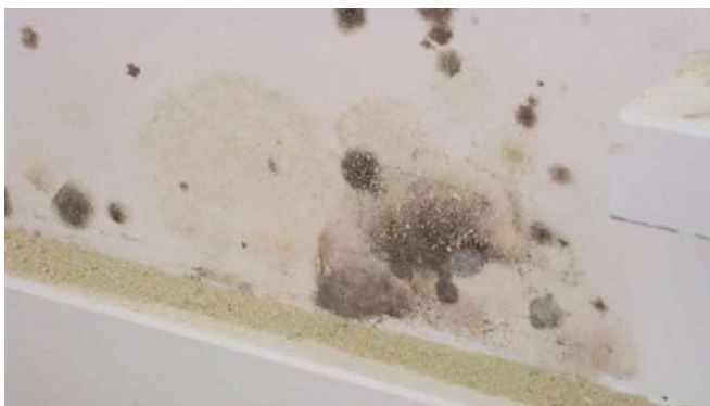
Internal mould growth.
