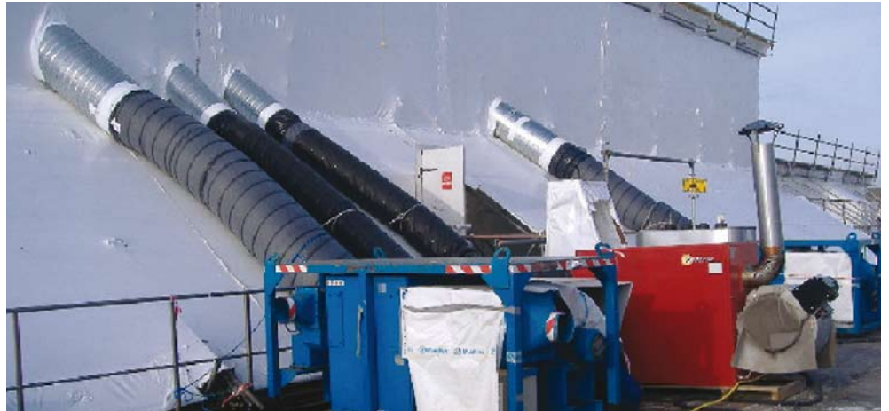
During repair the ship hull is covered by plastic foil to maintain a controlled climate. Dehumidifiers blow dry air into the covering, ensuring minimum corrosion between blasting away the old paint and applying the new.
