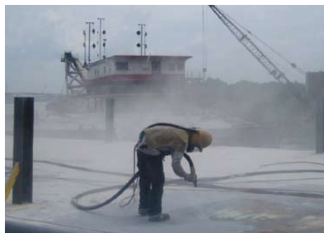
The use of Munters equipment allows ship repairs to be possible throughout the year.
