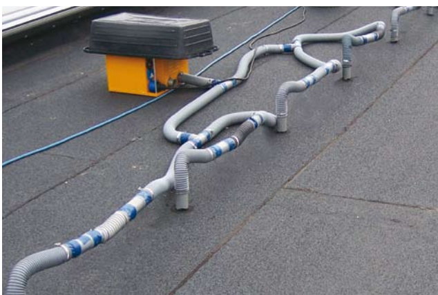
Drying solutions negate the need for expensive replacement.
