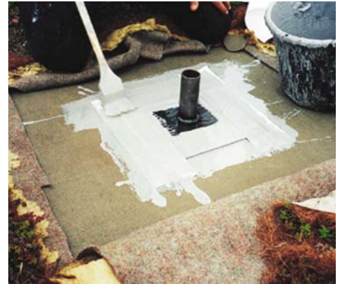
A targeted patch of damaged material.
