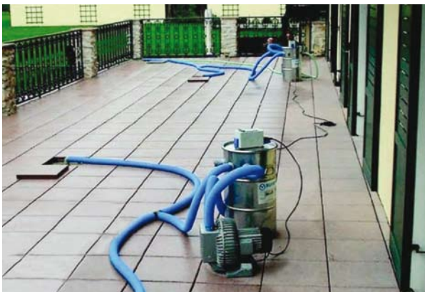
Drying an insulated terrace. As the wool is saturated, a water separator is connected between the terrace and the turbine.
