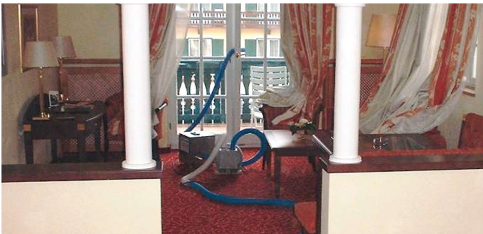
Lifting the carpet to drill just one hole ensures the entire insulation is dried with no damage to the expensive interiors.
