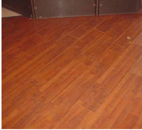
Damaged laminated floor.
