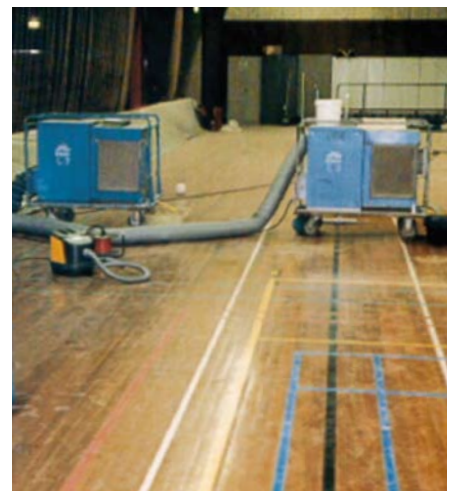
Dehumidification of sports floor.
