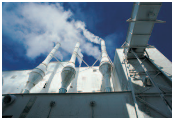
Stack rain separation units help to clean the emissions.
