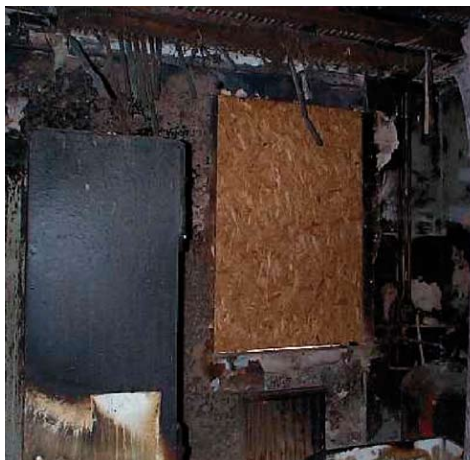
Extensive fire damage to bedroom before decontamination and refurbishment.
